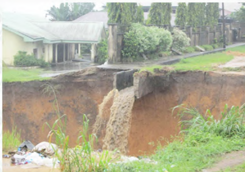
Plates 2a (above) and b (below): Section of gully sites at Ikot Nkebre showing failed roads and failed surface drains respectively.
