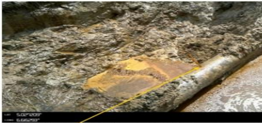
Close-up: 15mm drilled hole installed at 12:15 o'clock position on 14" at Edeoha. Picture was taken during Joint Investigati
