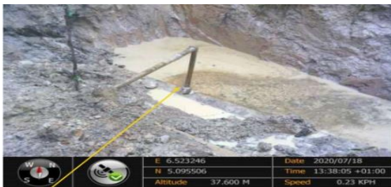
Close-up: Failed 2inch ball valve fittings installed at 12 o'clock position on 14" Okordia Rumuekpe Pipeline at Idu-Ekpeye. Picture was taken during Joint Investigation 18 th July 2020.
