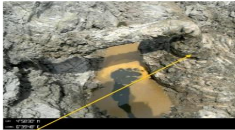
Close-up: 3" illegal valve with a concrete cast attached to a 3" galv on 20" Kolocreek -Rumuekpe Pipeline at Ihuowo. Picture was t 3rd October 2020.
