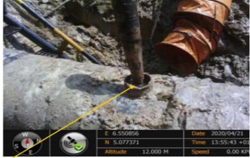
Close-up: 3" Nipple Installed at 12 o'clock position on Pipeline at Idu-Ekpeye. Picture was taken during Joint Investigation 21 st April 2020.
