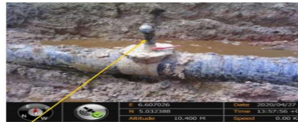
Close-up: 3" Valve Installed at 12 o'clock position on 14" Okordia Rumuekpe Pipeline at Edeoha. Picture was taken during Joint Investigation of 27 th April 2020.
