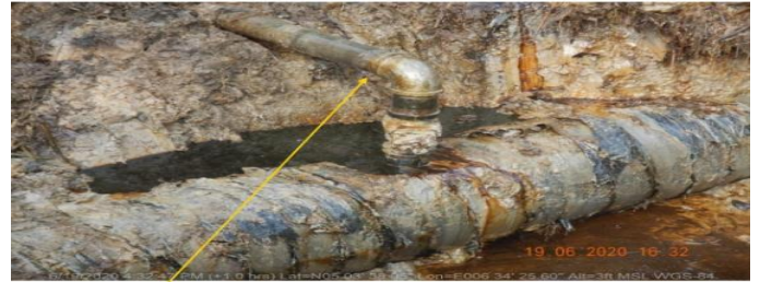
Closeup 1: Crude Oil theft point installed at 12 o'clock position on 14" Okordia Rumuekpe Pipeline at Ula-Okobo. Picture was taken during Joint Investigation 19th June 2020.
