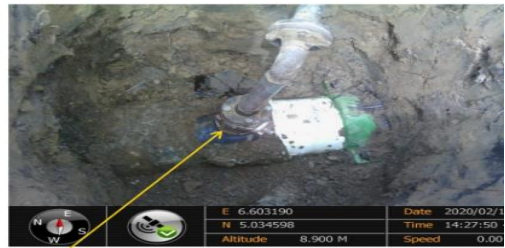
Close-up: Crude oil theft point installed at 12 o'clock position on 14" Okordia - Rumuekpe Pipeline at Ikata. Picture was taken during Joint Investigation of 13 th February 2020.
